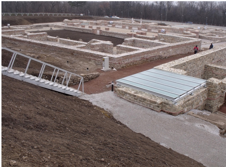
Fig. 21 — Novae. The Bishop's Complex in Novae after the Implementation of the EU Conservation Grant. View from South-East (Phot. A.B. Biernacki).
